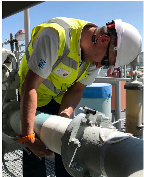
Installation on the air feed line.
