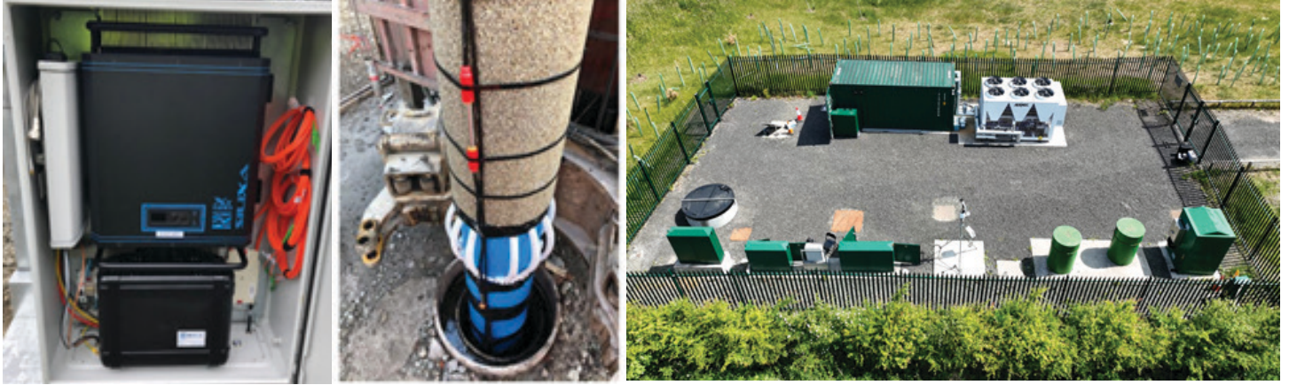
Figure 3 : Field deployment of the Silixa's XT DTS unit in an enclosure. (Centre) Fibre optic cable installation at a borehole in Glasgow observatory, (Right) Permanent infrastructure for heat and flow perturbations in a sealed, open-loop system.
